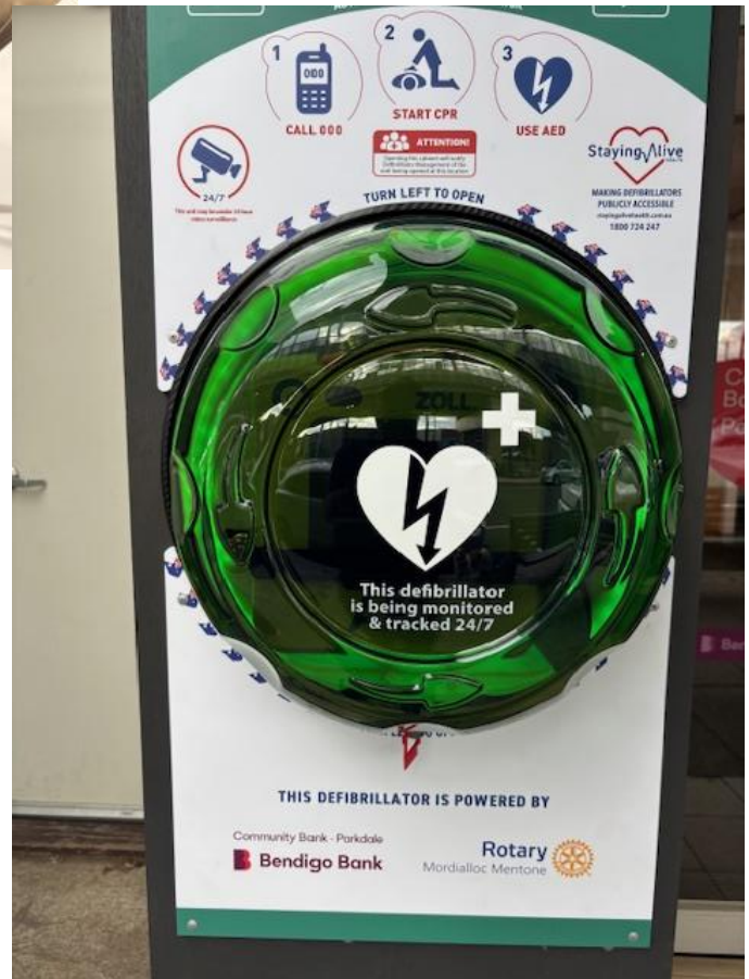
THE FIRST OF SEVERAL DEFIBRILLATORS TO BE INSTALLED – TTHIS ONE OUTSIDE BENDIGO BANK PARKDALE
